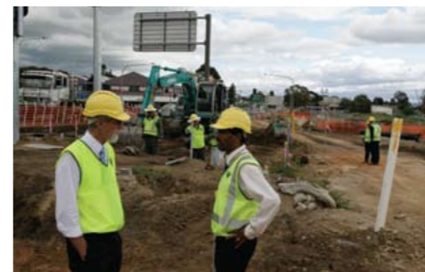
RTA staff Geoff Fogarty and Vasee Vaseeharan inspecting work on the Narellan Road extension.
