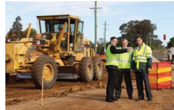
Left to right – Minister for Roads Eric Roozendaal, Liverpool MP Paul Lynch and Macquarie Fields MP Andrew McDonald inspecting work at Cowpasture Road, June 2008.
