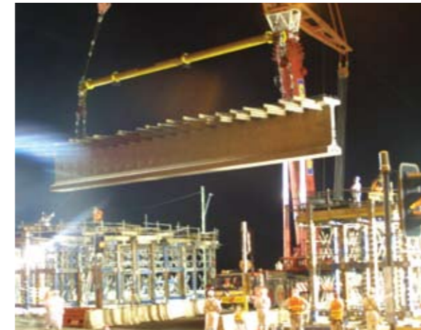
Night works: Erection of the bridge girders over Weakleys Drive Interchange, June 2008.
