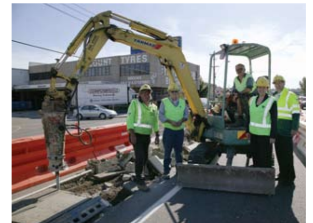
Buses get a green light: Left to right – Team Leader Ken Collins, Work Supervisor Geoff Cam, RTA contractor, with Member for Parramatta Tanya Gadiel and Minister for Roads Eric Roozendaal at Parramatta.
